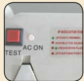
Not Illuminated = Emergency Mode
